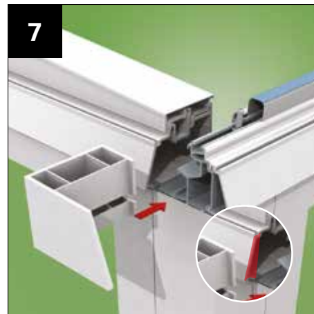
'Butter' with silicone then slide the eaves beam end cap block into place. It will be necessary to silicone seal the area highlighted in the inset image.
